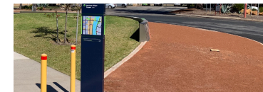
Cracked pea gravel for verge refresh to Minson Ave
