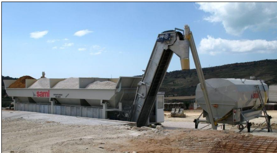
Photo 3: Dry mix plant
