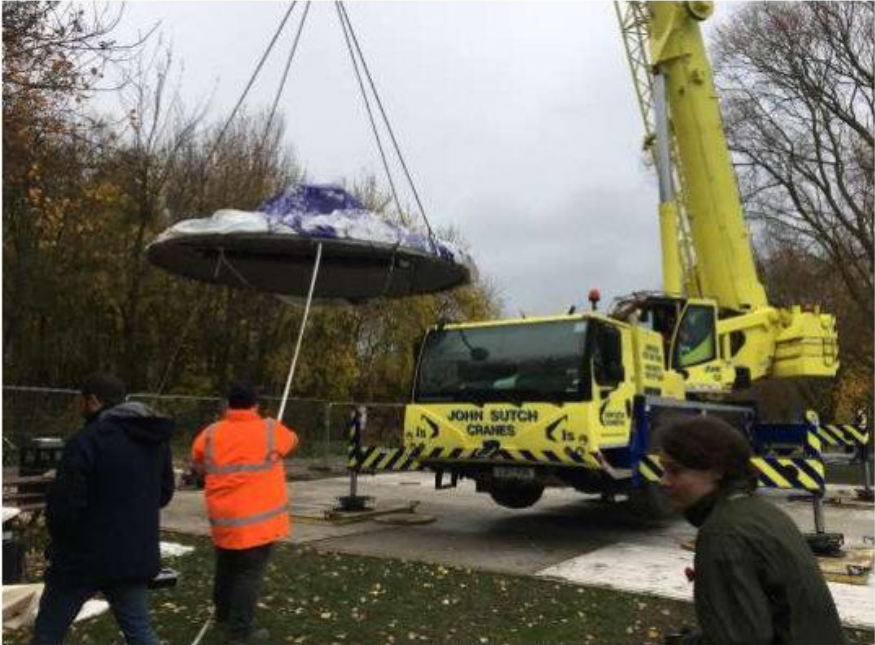
Artwork is then lifted into the water, using the crane or a telehandler. The telehandler needs a reach forward of 4m+.
