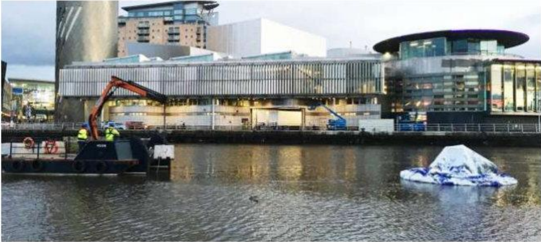
Alternatively, the concrete mooring can be placed into the water with a barge.
