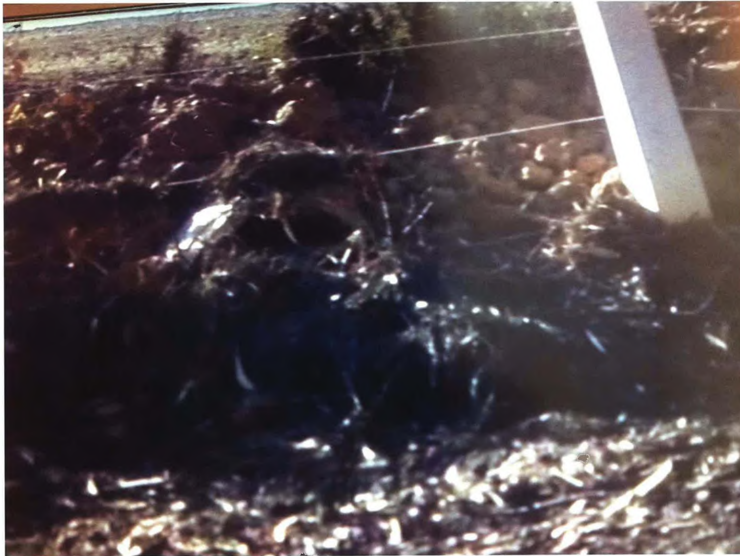
TAKEN 15.4.2018 DEBRIS ON FENCE ALSO BLOCKING CULVERT
