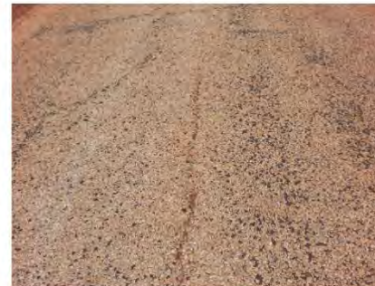
Existing issues: Surface Age
